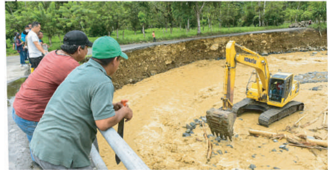
De manera prioritaria se atendió la emergencia invernal por la crecida del río Limón, en Bucay. Priority was given to the winter emergency caused by the flooding of the Limón river in Bucay.
