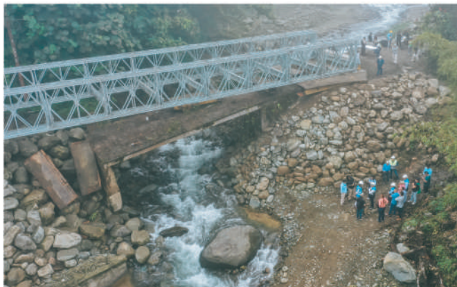
Se han instalado 18 puentes Bailey, que sirven para unir a comunidades Eighteen Bailey bridges have been installed, which serve to link isolated communities.
