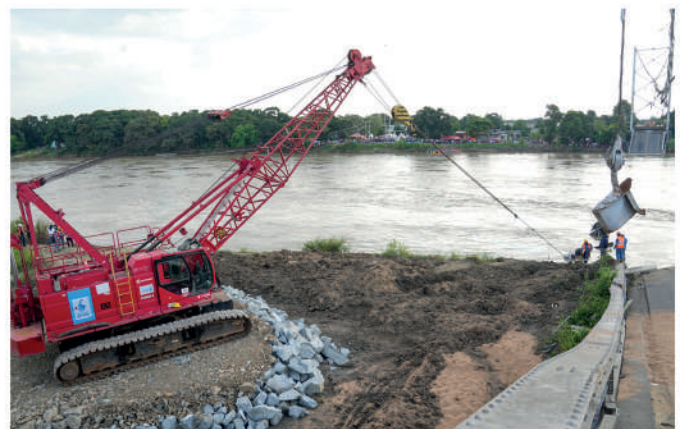
El puente estaba asegurado y su reposición corre a cargo de la concesionaria. The bridge was insured and its replacement is the responsibility of the concessionaire.
